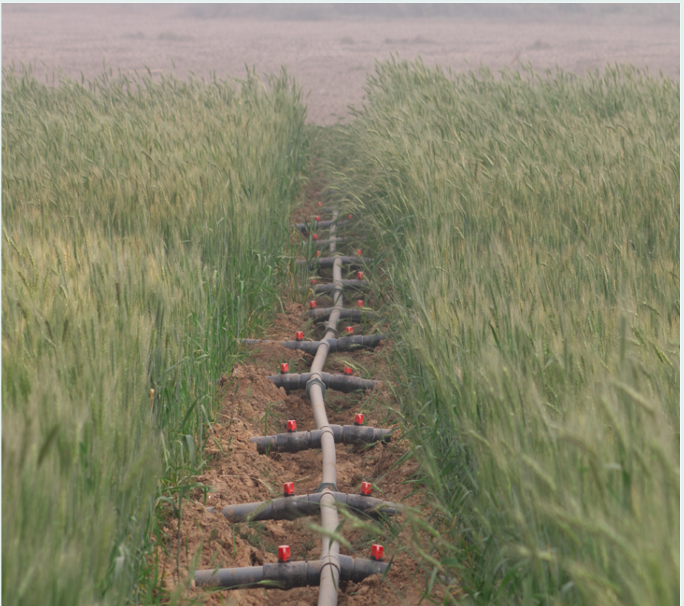
A modern pressurized water conveyance distribution system in demonstration site in Alkamawah, Kano State, Nigeria.
