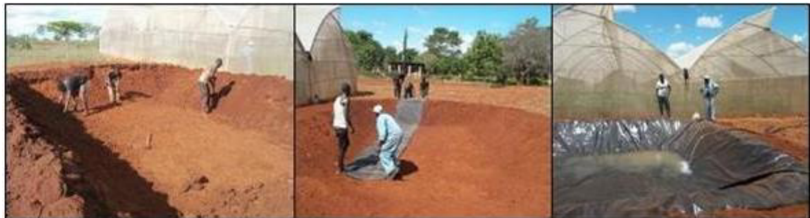
Establishing a small fishpond (left to right): 1) excavating and smoothing the pond, 2) spreading the PVC liner and burying the edges, and 3) filling the pond
