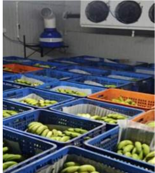
Industrial ripening chamber with refrigeration and gas control (Credit: Nilkamal)
