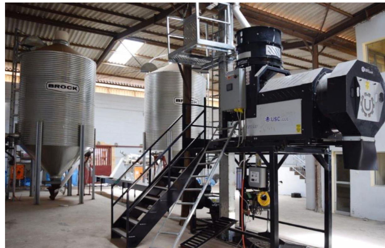
Equipment needed to produce Aflasafe® at commercial scale.
